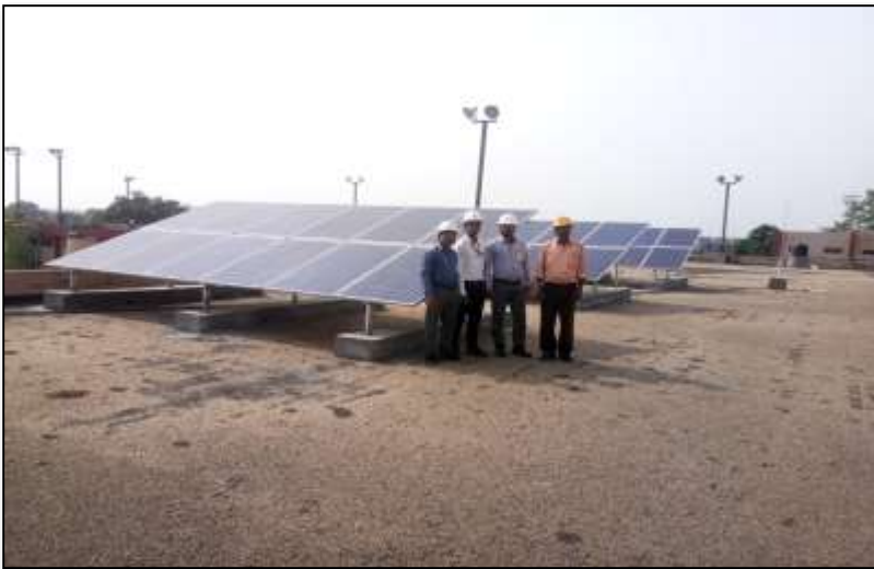
Solar PV Plant in DM Plant.
