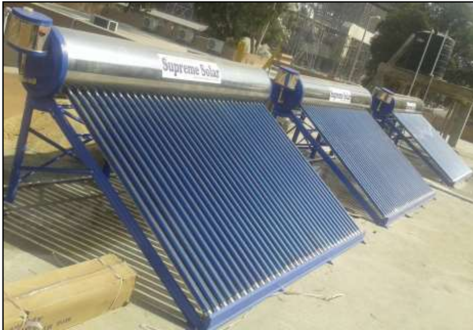
Solar Water Heater at Plant
