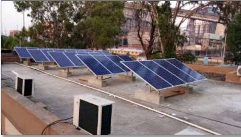
Solar PV Plant in Canteen.
