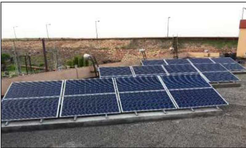
Solar PV Plant in Ash Pond.
